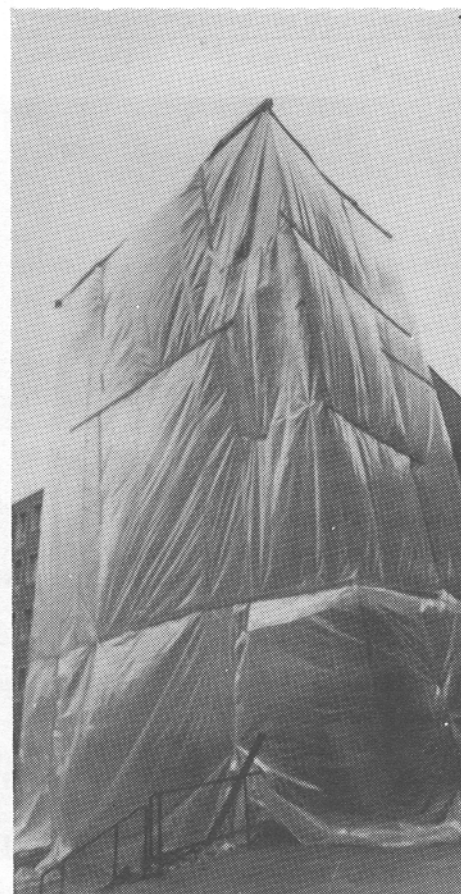
The new elevator under construction in Graham Hall will improve accessibility for disabled students.
