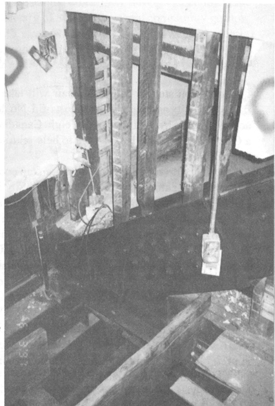
A splintered wooden truss in Room 413 of Wesley Hall had to be clad in steel.
