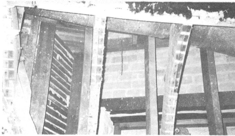
Behind Wesley's walls, extensive structural damage was apparent.
